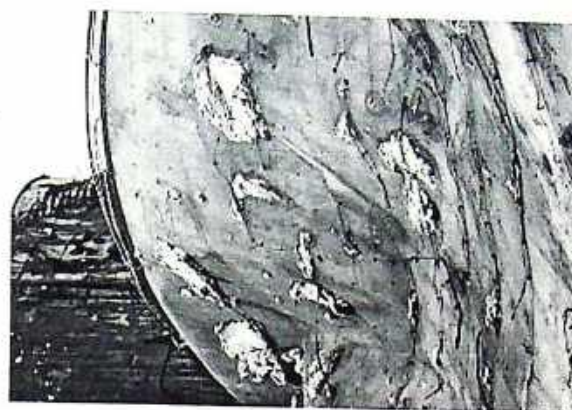
Destroyed oil tank at Novi Sad
