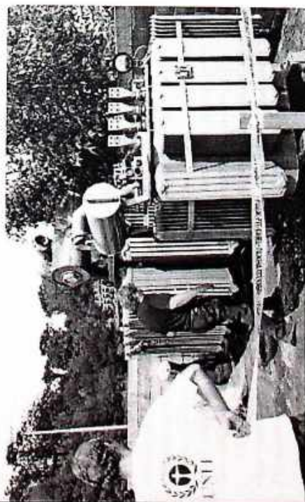
Inspection of damaged transformers
